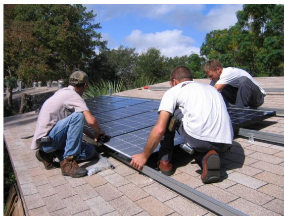
Figure 1. Installation of the 3.85 kW solar photovoltaic (PV) system at the existing home case study. (Source: University of Florida)
